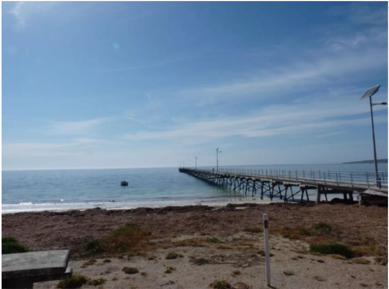
THIS JETTY WAS ONCE PART OF A VITAL TRANSPORT HUB FOR THE REGION.
